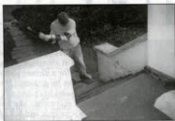
David Marino of Van-Go Contracting beginning to demolish the old cement front porch.
